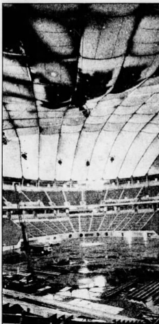
Staff Photo by John Croft Snow made a visible bulge in the dome Thursday as light streamed through the translucent material. Water from the melting snow accumulated on the field below.
